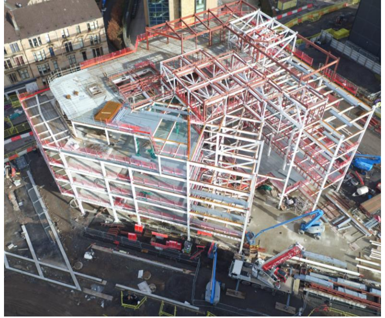
The steel frame of the Clarice Pears Institute of Health & Wellbeing nears completions
