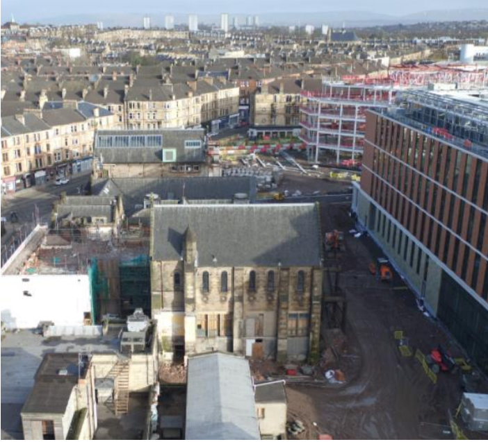
The Alexander Elder Memorial Chapel will be retained as surrounding buildings are demolished
