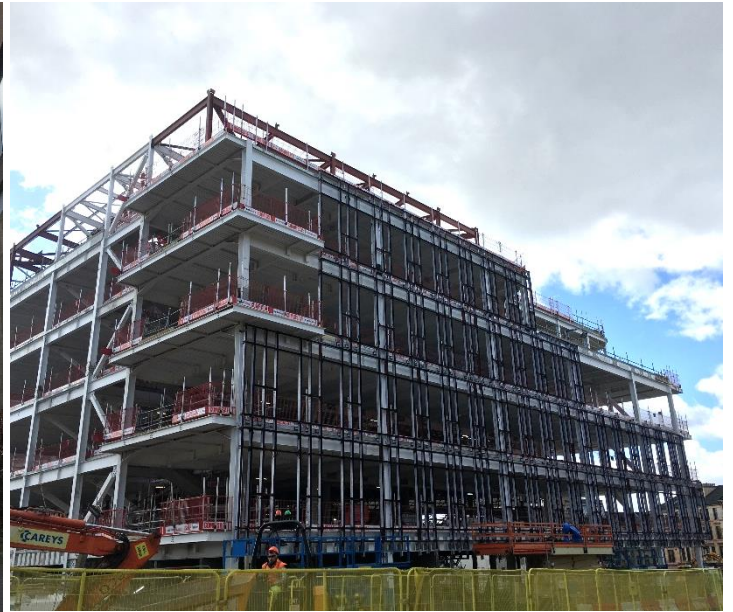
The envelope works underway at the Clarice Pears Institute of Health & Wellbeing
