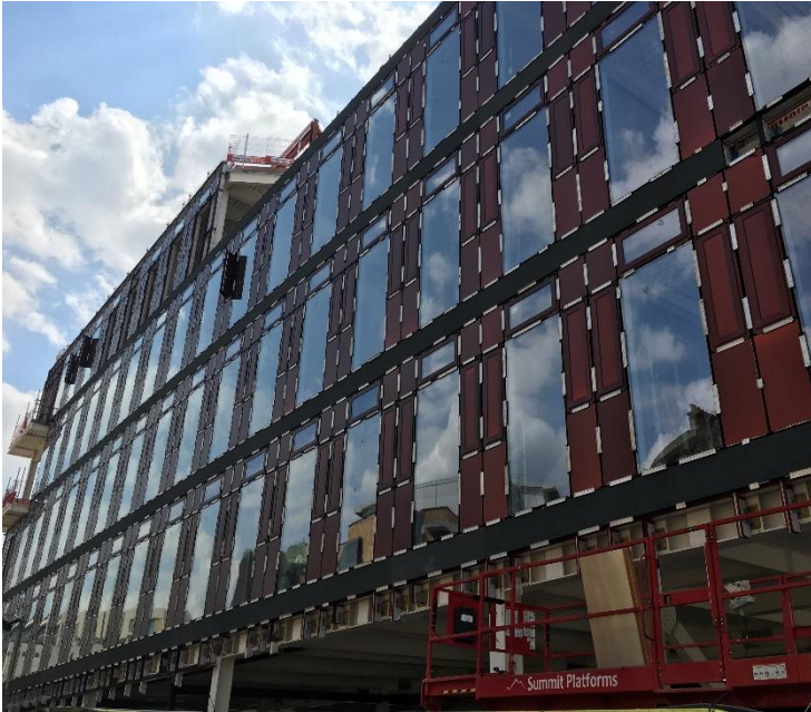
Envelope works ongoing at the North elevation of the Clarice Pears building
