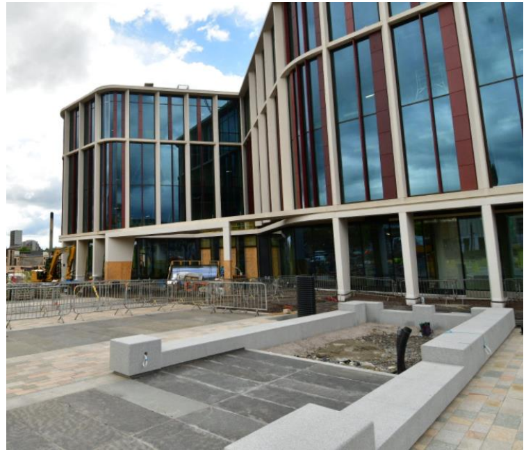
Public realm and landscaping works on University Square outside the Advanced Research Centre
